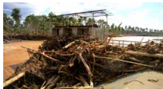
Silted dam of Ngan CIS, Compostela Valley during landfall of typhoon Pablo on December 4, 2012.
