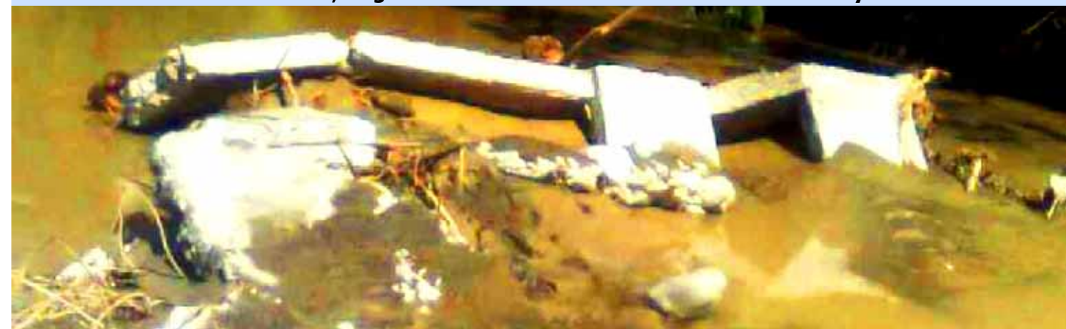
Diversion Structure (Intake) of San Pedro CIS, Caraga, Davao Oriental washed out during the Typhoon Pablo land fall at Davao Oriental on December 4, 2012. Photo courtesy of Engr. Jimmy J. Ceros, Acting Davao Oriental IMO.
