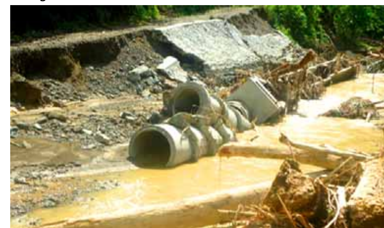
Damaged Road Crossing and Protection Dike at Nuevo Iloco CIS, Mawab, Compostela Valley during Typhoon Pablo's landfall on December 4, 2012.
