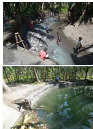
Cabacungan CIS Protection dike on-going repair by IA(upper photo); completed protection dike (lower photo)
